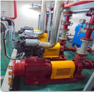
Trạm bơm chữa cháy/ Fire pumping stations
